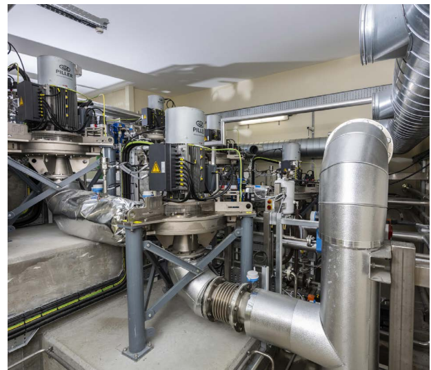
MVR equipment, including three PILLER VapoFans
